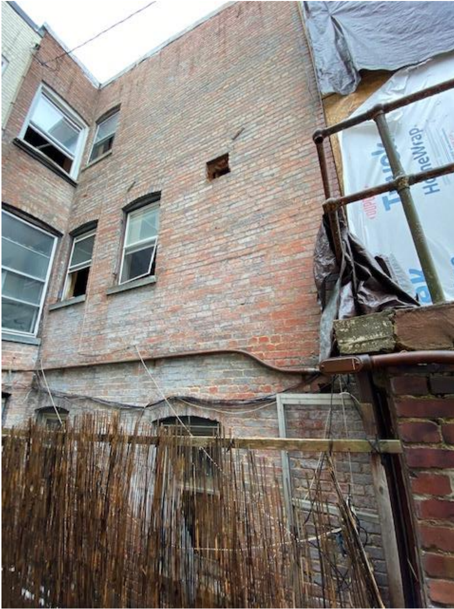
Back windows wide open and unsecured.
