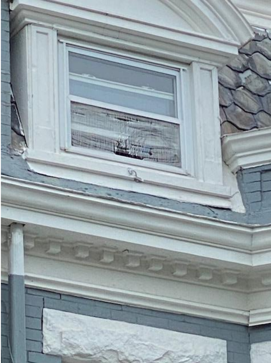
The front third floor window is unsecured.
