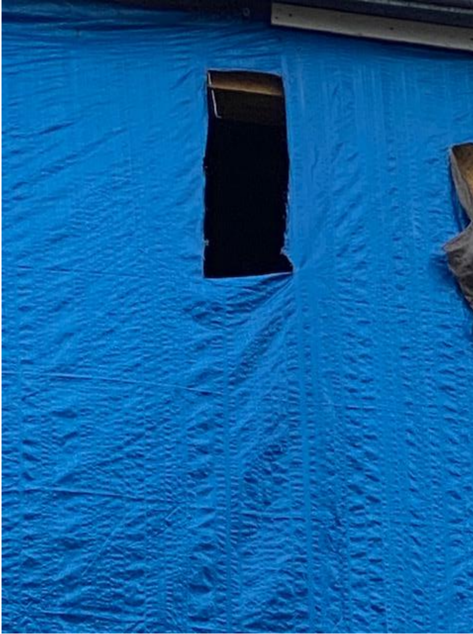
This is the tarp that covers the back wall. The second floor is completely open as shown by the hole in the tarp.
