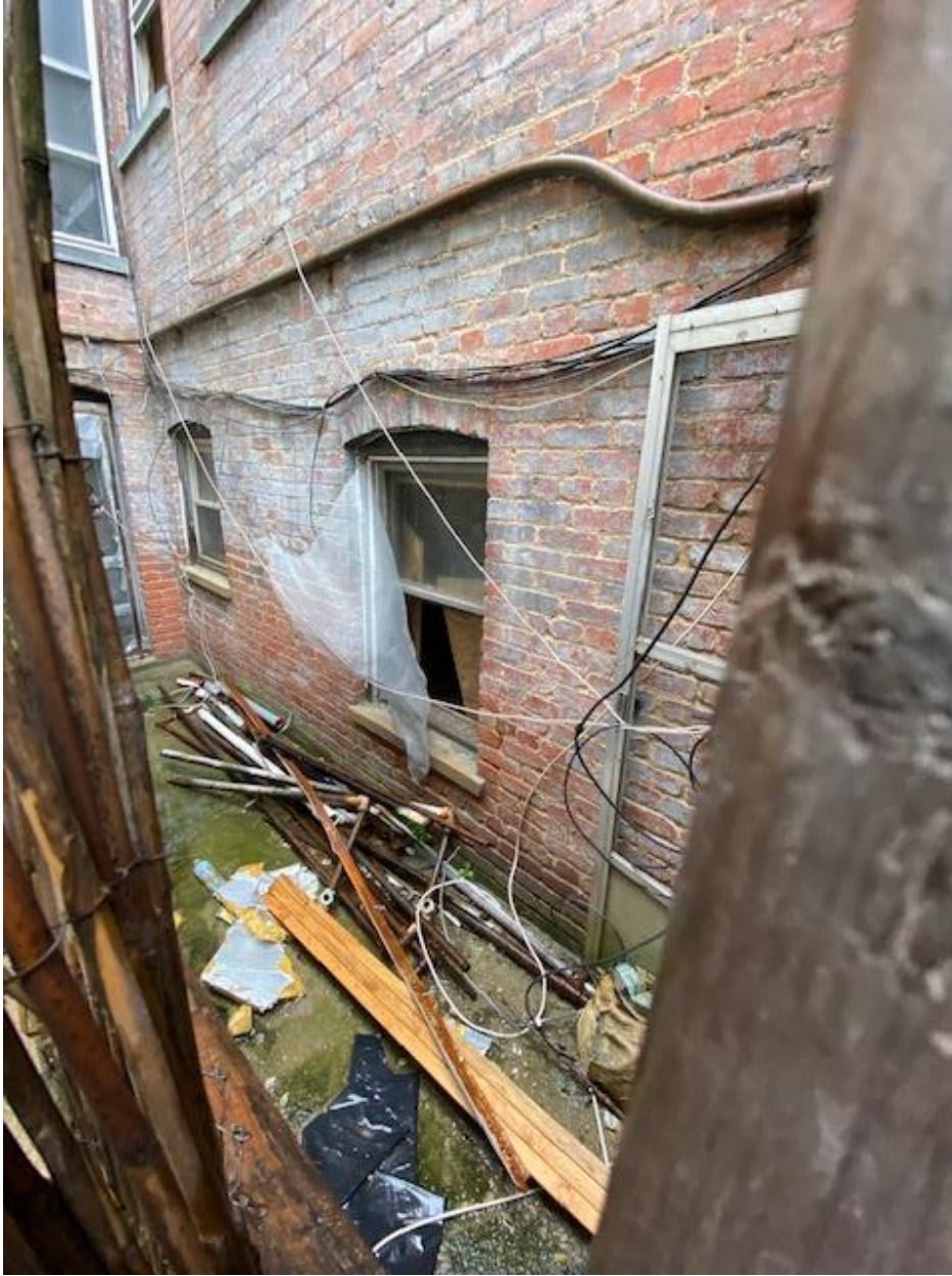
Ground floor window open and unsecured. Construction debris littering the ground. Providing nesting to rats and termites.
