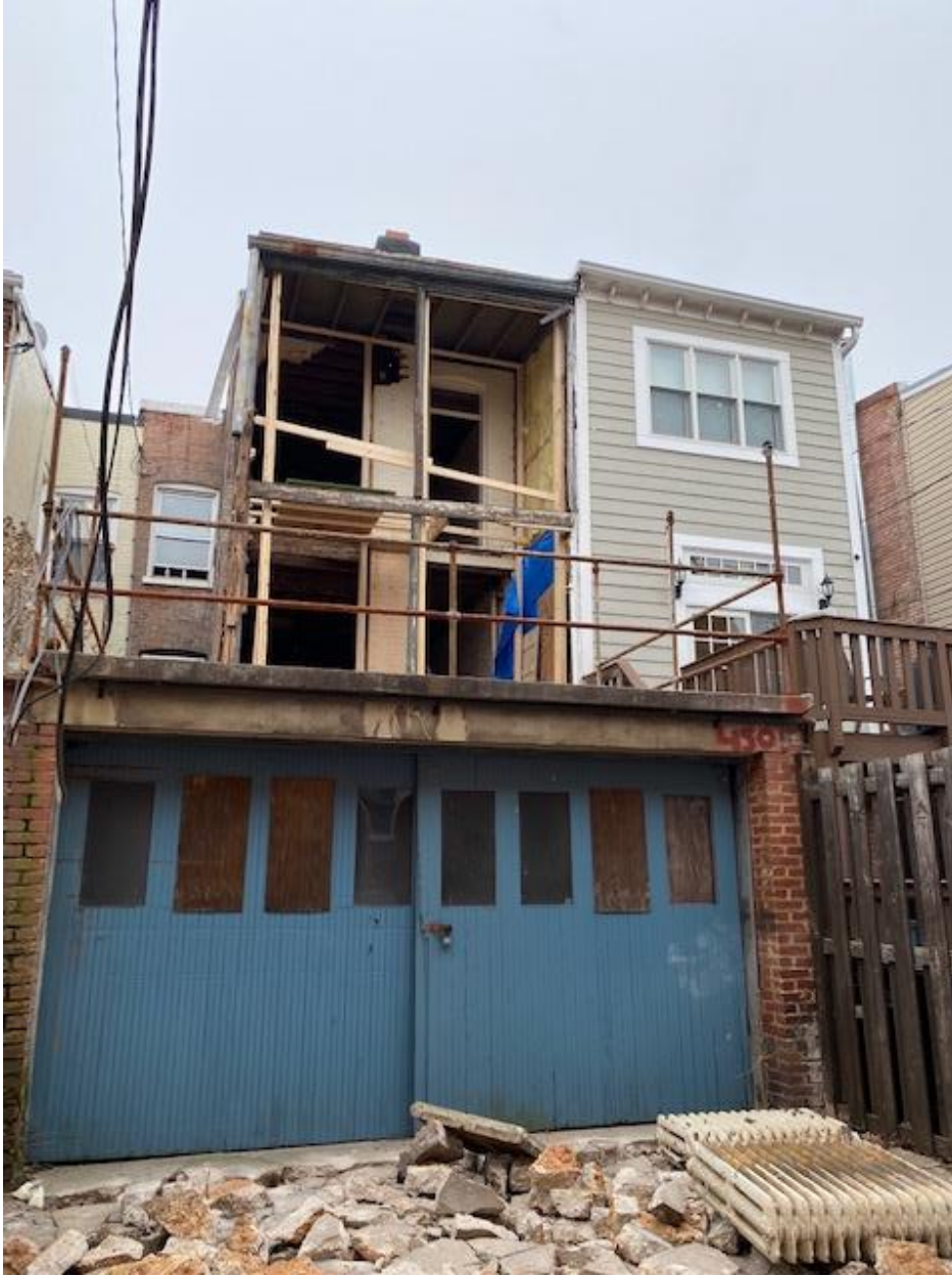
The back wall of the house was completely removed which exceeded the scope of the original permit.
