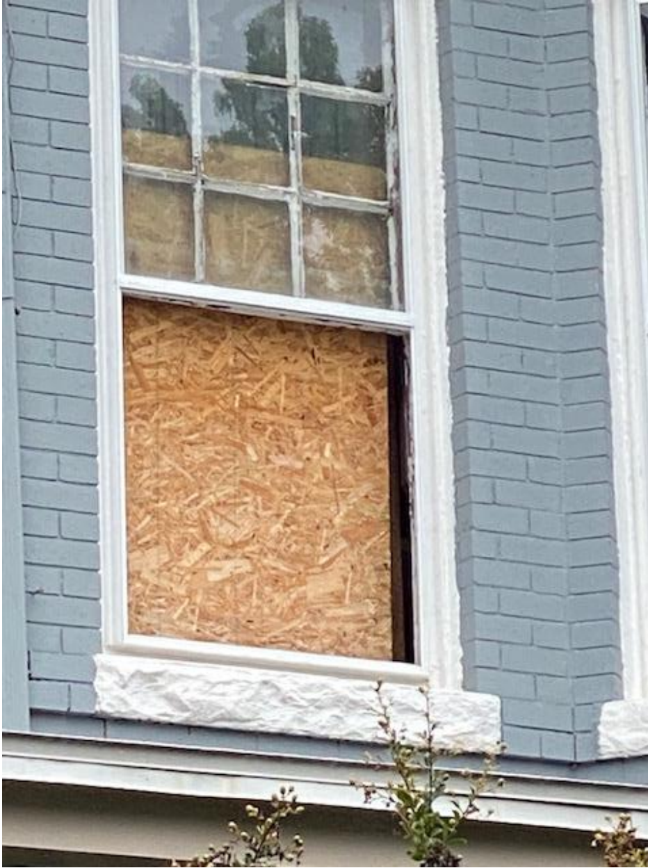
The front second floor window is unsecured.
