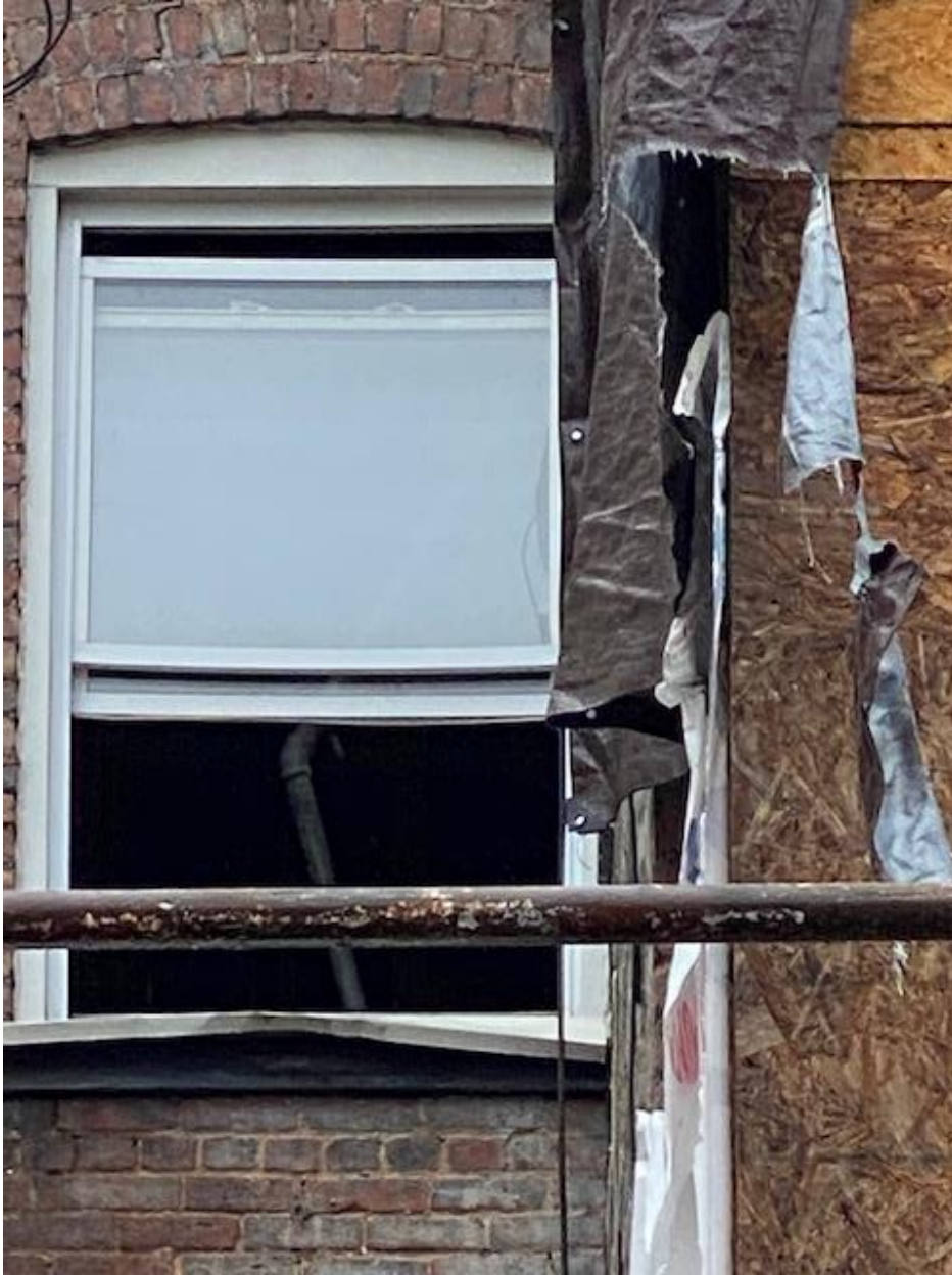
Window in the back open and unsecured.
